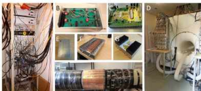
Figure 2: A) 19" rack in equipment room containing power supplies, control and supervision computers, modulators, and control electronics; B) Modulator cassette for 2 channels; C) LDMOS power amplifier; D) 16 amplifiers in rack directly at the back side of magnet; E) 32-ch receive chain switch; F) 2nd-stage receive amplifiers; G) magnet room PIN diode power supply for body coil; H) integrated 32-ch body coil.
